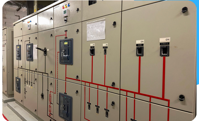
Example of Distribution Board
