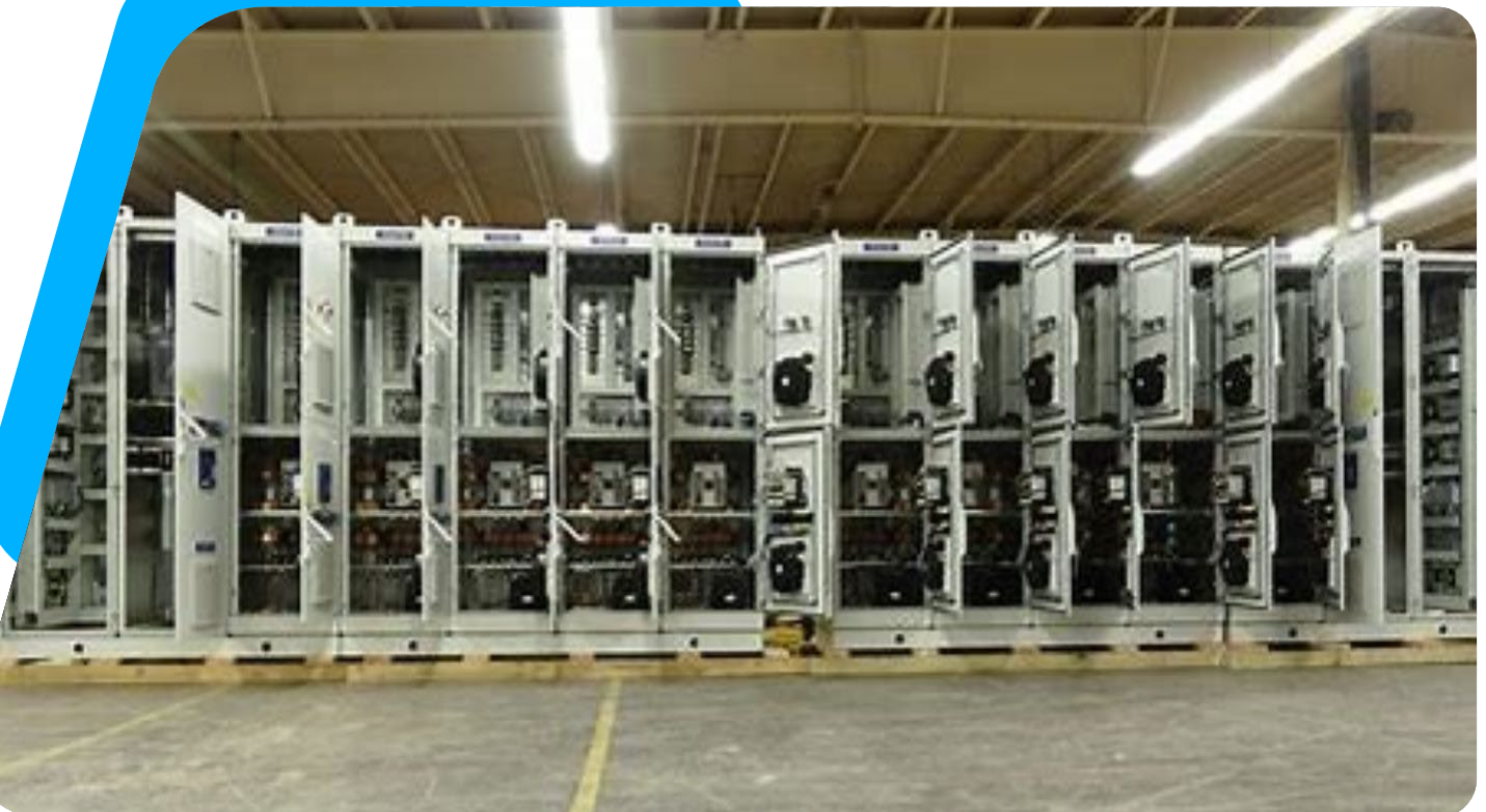
Design, Manufacture and Assembly of Electrical Cabinets
